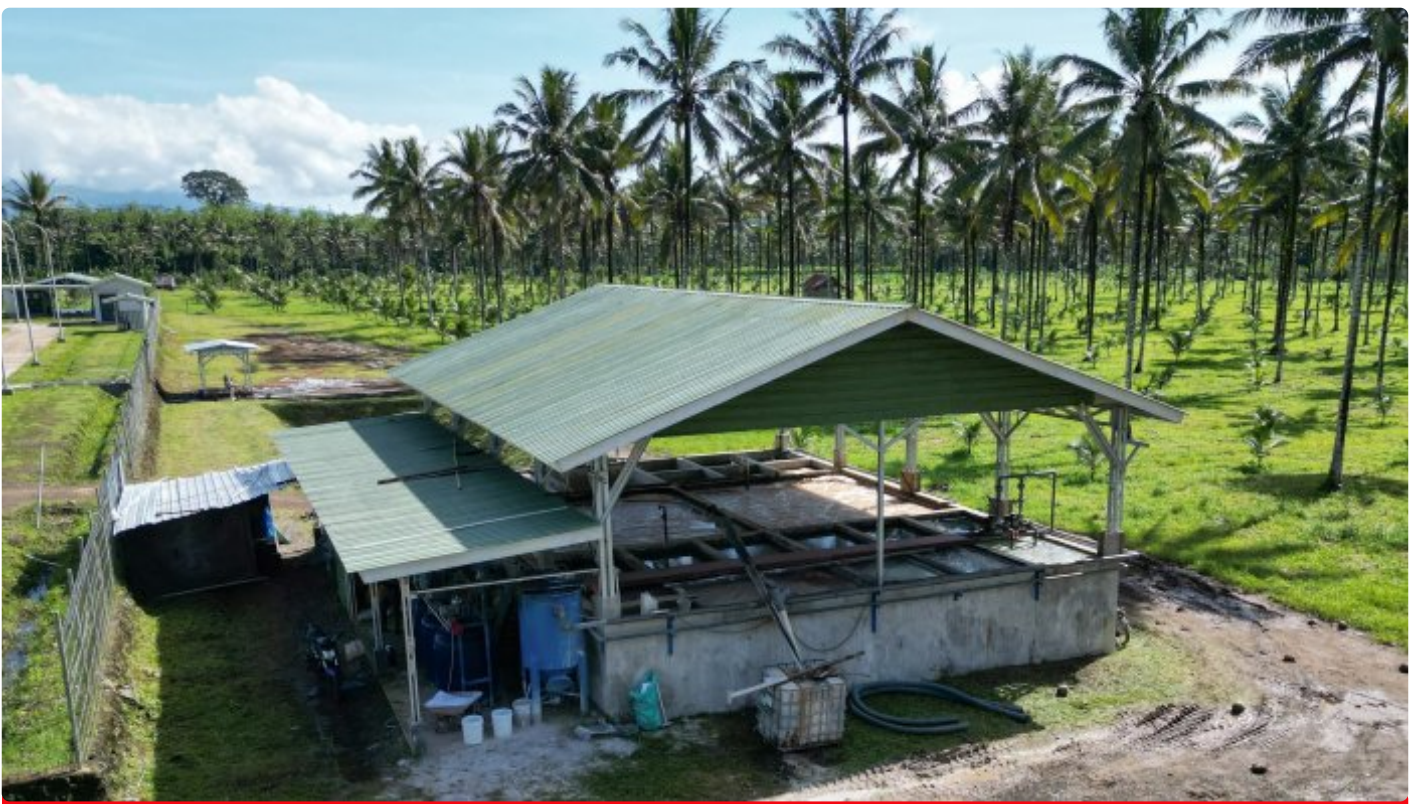
Dewacoco Waste Water Treatment Plant (WWTP)
